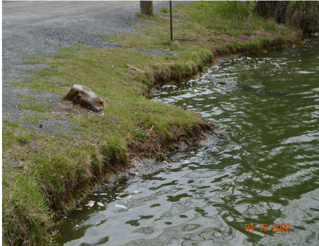
Eroding shoreline at the South Gate pond
